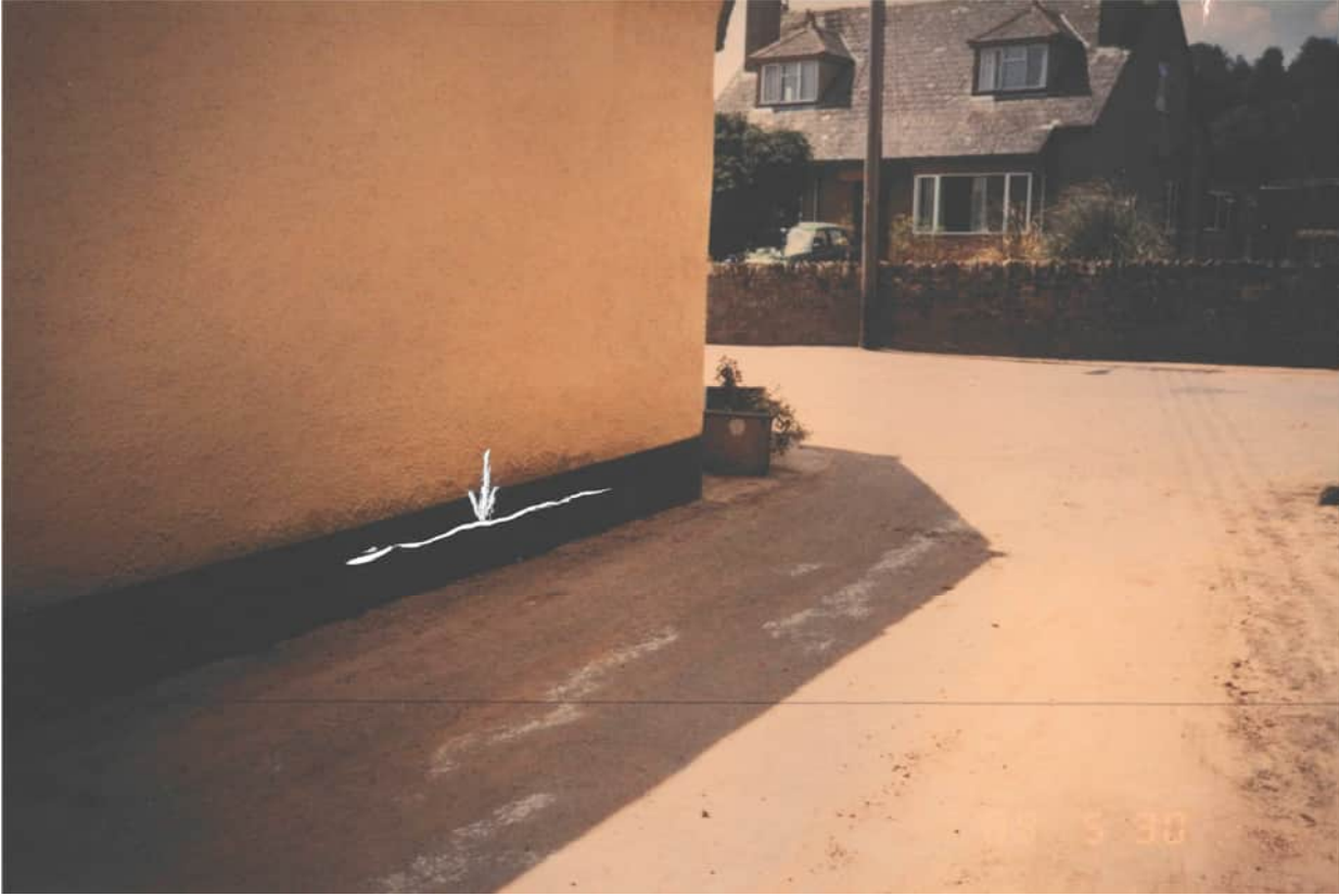
Brook House, the road in the foreground is the preferential route for excess flows
